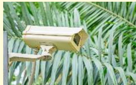
24 hrs. Security with CCTV
